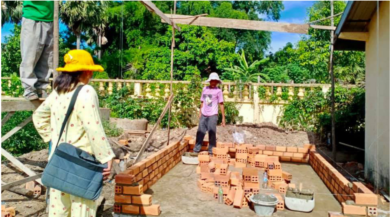
Good Shepard Conference, Cambodia, building school latrines as part of their Good Works Program.
